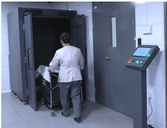
Clean linen inbound scanning performed through a high-density RFID cabinet
